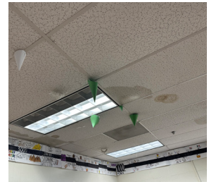
Boiler room leak on classroom ceiling at Oxford Academy
